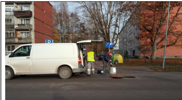
Jurmala_section A_Kauguri district_installation of automatic sampler with a level sensor in the storm water manhole
