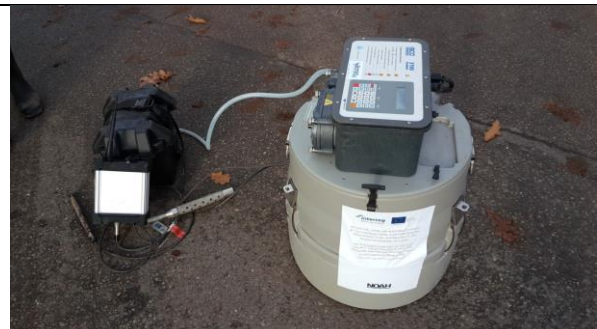
Jurmala_section A_Kauguri district_installation of automatic sampler with a level sensor in the storm water manhole
