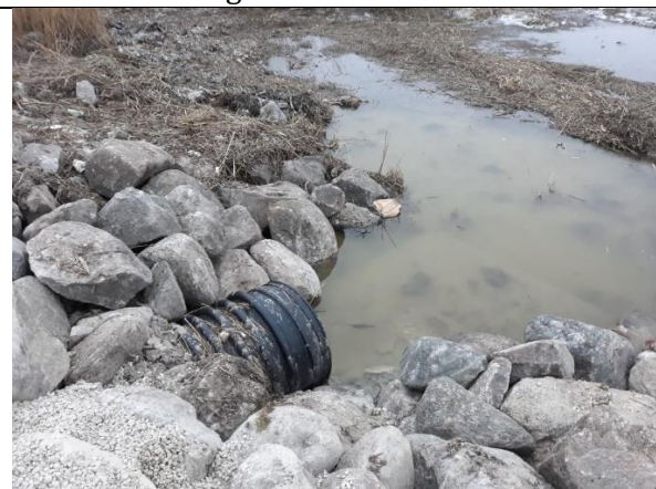
Outflow to Haapsalu bay
