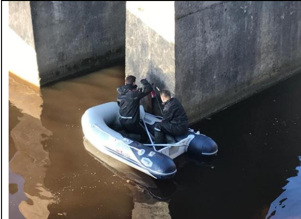
Instalment of automatic hydrological stations
