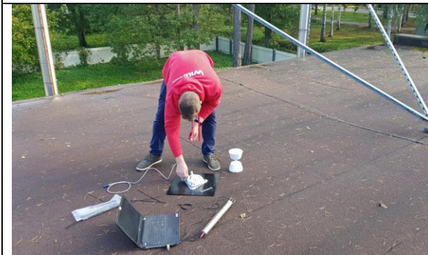
Jurmala_section B_Melluži district_installation of local meteorostation on the rooftop of sewage pumping station
