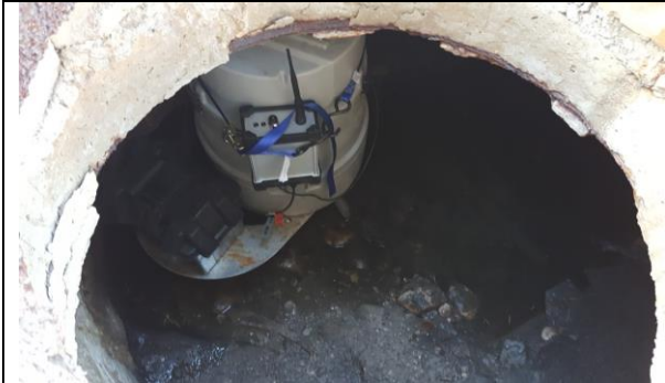
Jurmala_section C_Dzintari district_installation of automatic sampler with a level sensor in the storm water manhole
