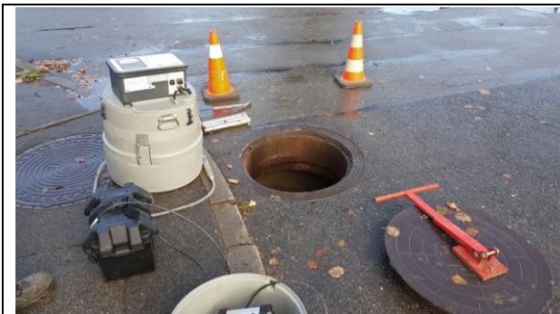
Jurmala_section B_Melluži district_installation of automatic sampler with a level sensor in the storm water manhole
