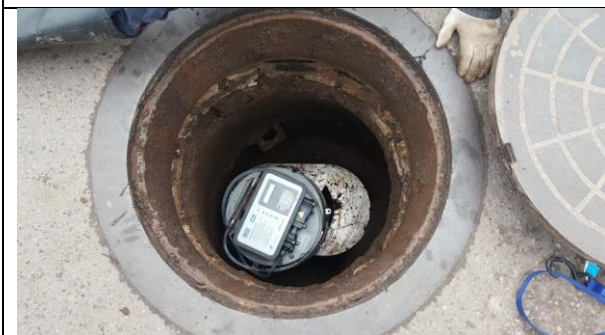
Jurmala_section A_Kauguri district_installation of automatic sampler with a level sensor in the storm water manhole
