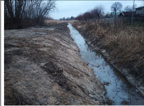
Preparing site for installment of the RTC, deepening inflow ditches and removal of the reed in the proximity of the weirwall base
