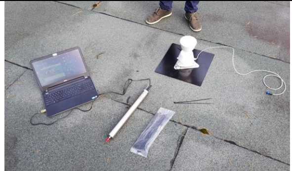
Jurmala_section C_Dzintari district_installation of local meteorostation on the roof of Jurmalas udens Ltd warehouse
