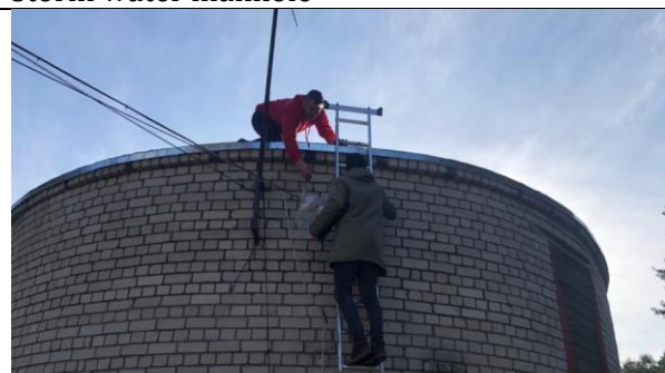
Jurmala_section A_Kauguri district_installation of local meteorological station on the rooftop of sewage pumping station
