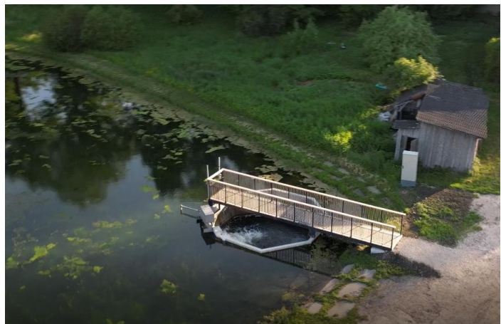
Smart Weirwall System (SWS) in Rakvere, Estonia.
