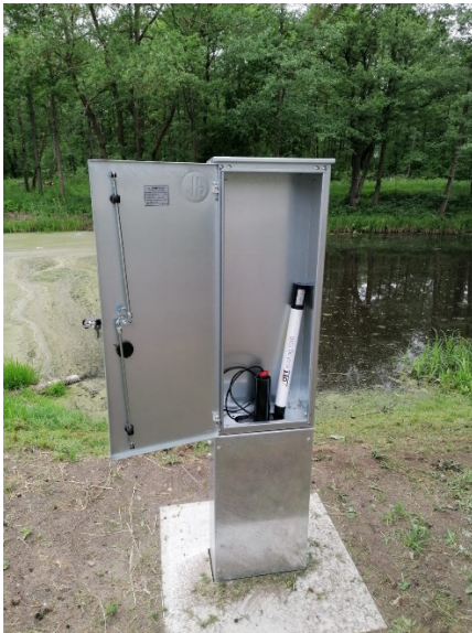
Picture 1. Water level sensor installation in Liepaja, Latvia.
